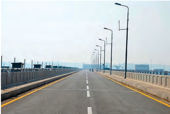
> Figure A7: New road connectivity. The 1.34-kilometer bridge across the New Khanki Barrage connects the opposite riverbanks.
