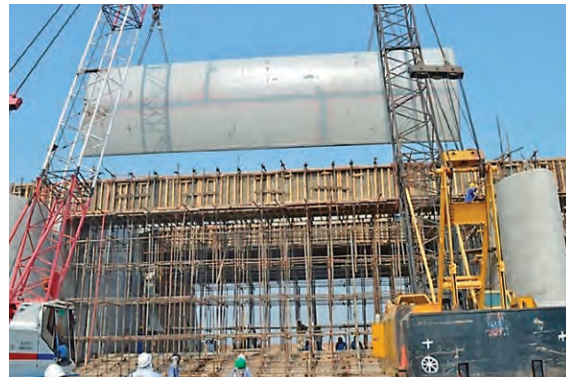
➤ Figure A4: Gate installation. Gate being installed in one of the bays.
