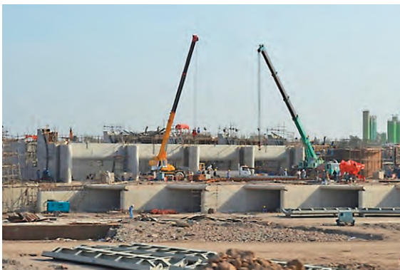
➤ Figure A5: Silt excluder under construction. Removing the silt from the river to divert clearer water to the canal.
