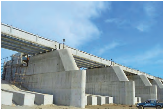
➤ Figure A3: Barrage bays under construction. The New Khanki Barrage has 65 bays.
