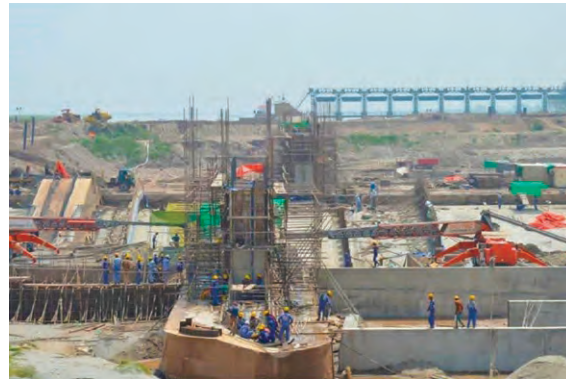
➤ Figure A2: New Khanki Barrage project site. Work continued while the old headwork, as seen on the right, was still operating.
