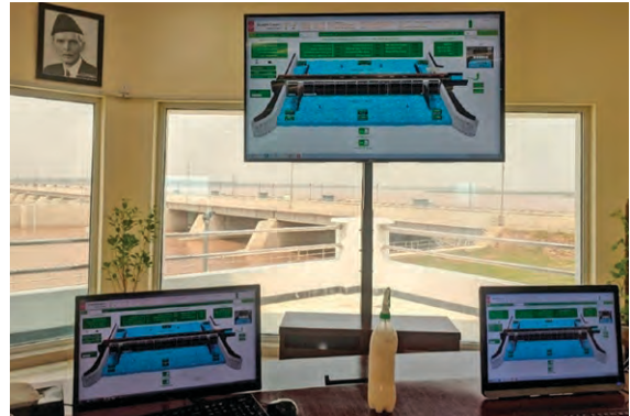
> Figure A8: Supervisory control and data acquisition system. The view from the control room, with the barrage in the background.
