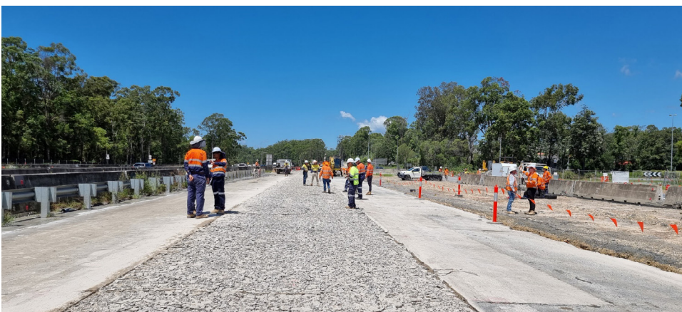
Figure 21 Coal ash fill used instead of earth or rockfill at Kangy Angy
