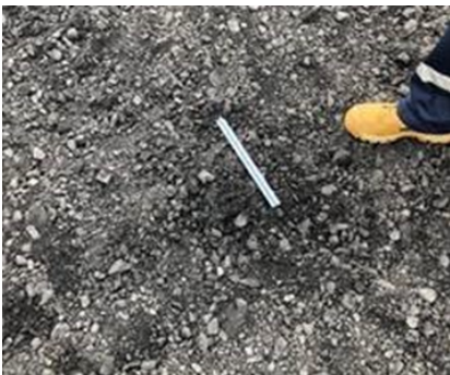
Figure 20 Granular Coal Wash Rejects at R31 Drainage Layer
